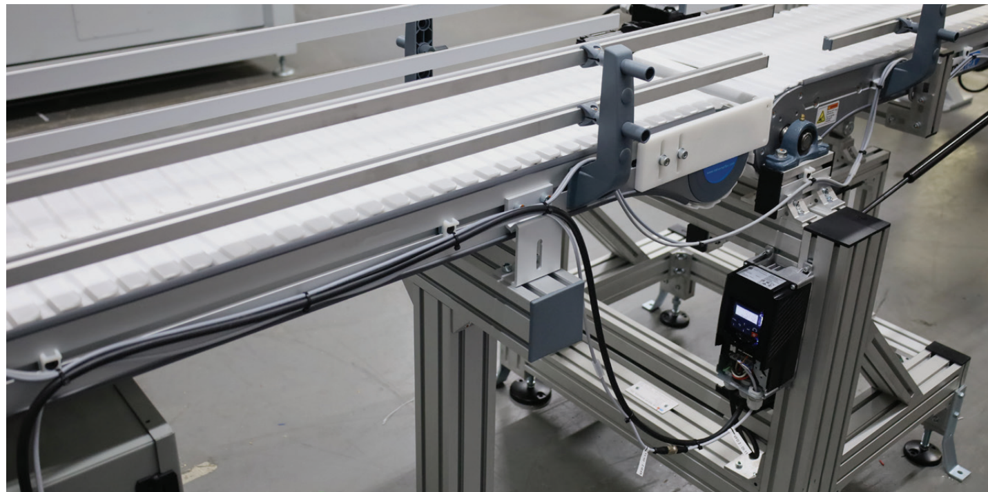
In this VersaFlex example, two conveyors meet up, with the one on the right side being a lift gate which allows for line access.
