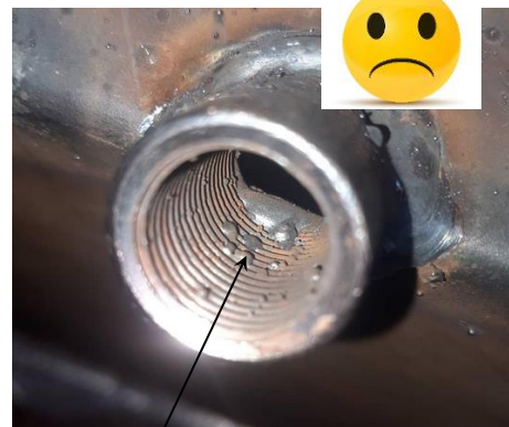
Excessive weld spatter
