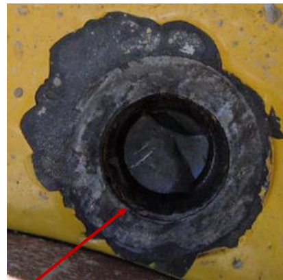
Fatigue failure of the bolt after the breakdown of the paint film at the joint interface
